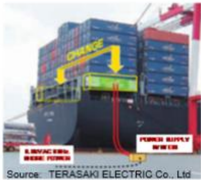
Onshore power supply to ships at berth Source: TERASAKI ELECTRIC Co., Ltd
