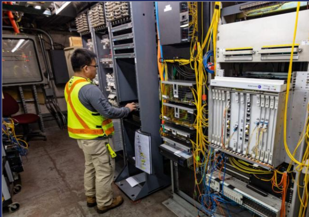
Upgraded Signal System
