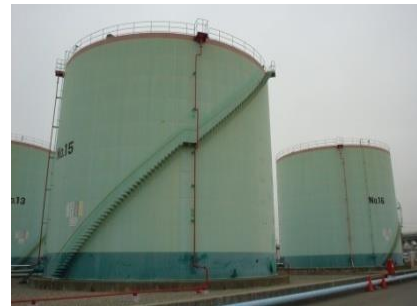
Warehouses for Hazardous Goods
