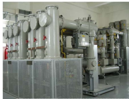
Gas Insulated Switchgear
