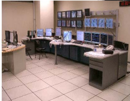
Station Control Room
