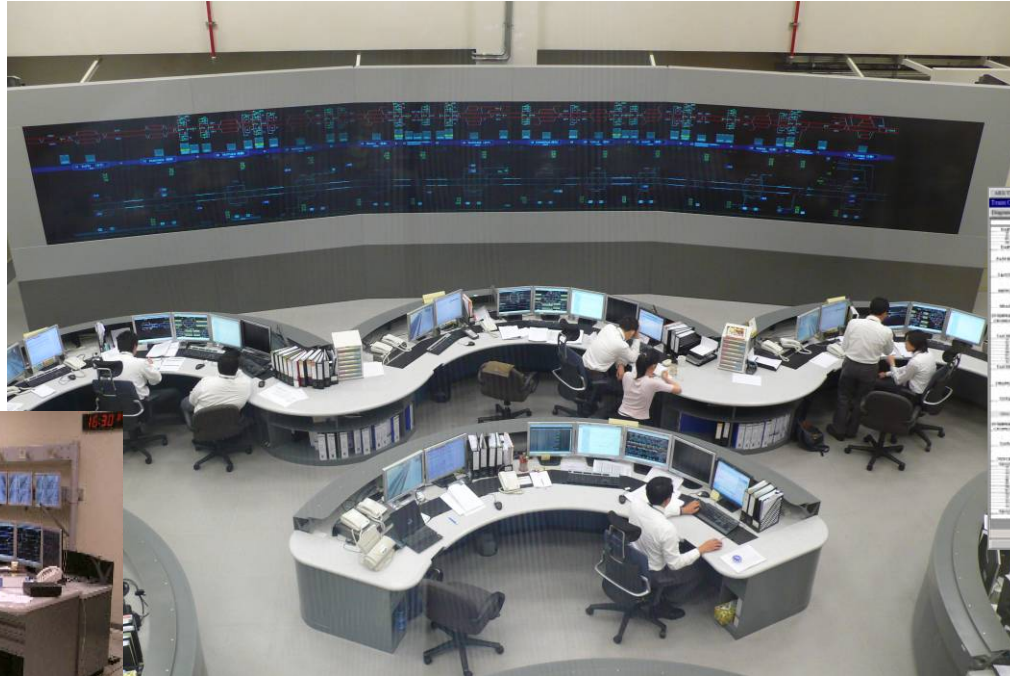
Operation Control Center
